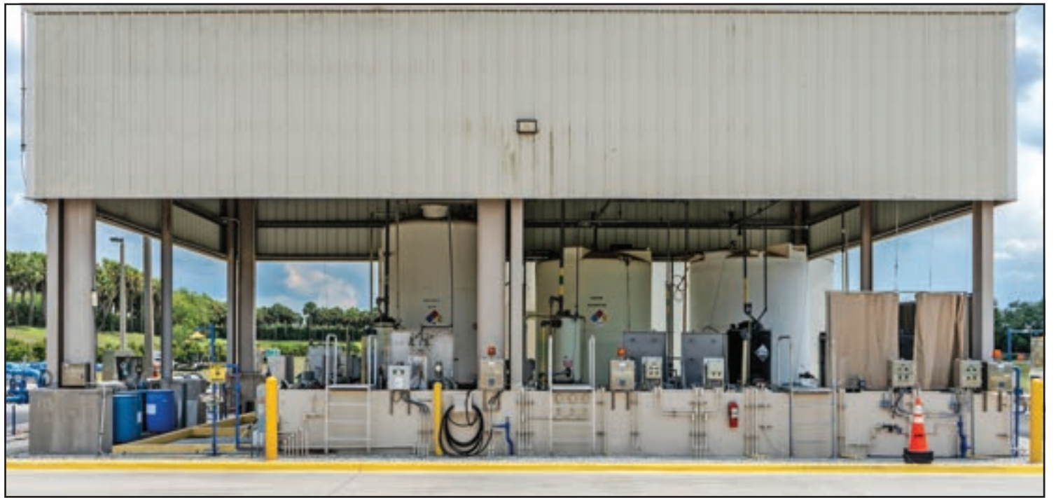
The AMUC water treatment plant is equipped with cutting-edge filtration systems, direct aquifer pipelines and ultrafiltration technologies.
